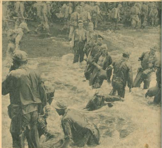
8—ROAD-BUILDERS. You'd never guess it, but these Gyrenes are laying a sandbag road under a rough three-foot surf so trucks, bulldozers and other heavy engineer's equipment can drive to beach from LSTs offshore.
